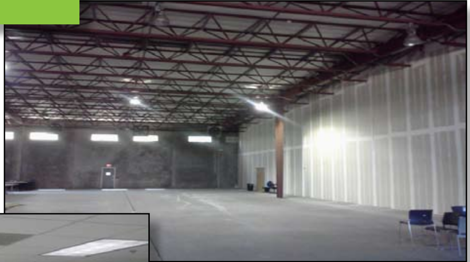
Warehouse Area 20' Eaves Sprinkled
